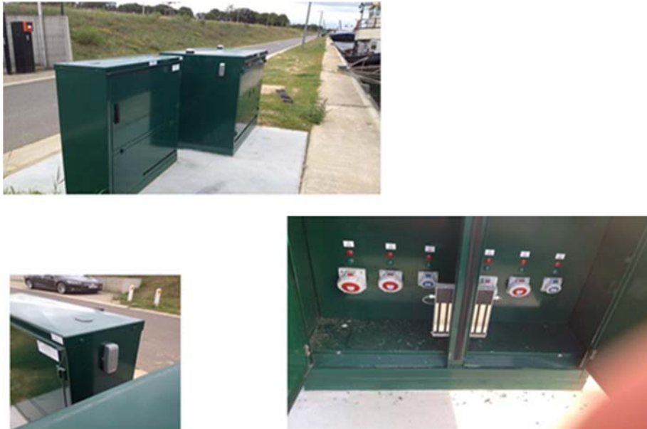
Figure 5. Shore power installations in the waiting port of Wijnegem
